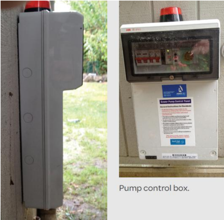
Figure 14 – Pump control box
