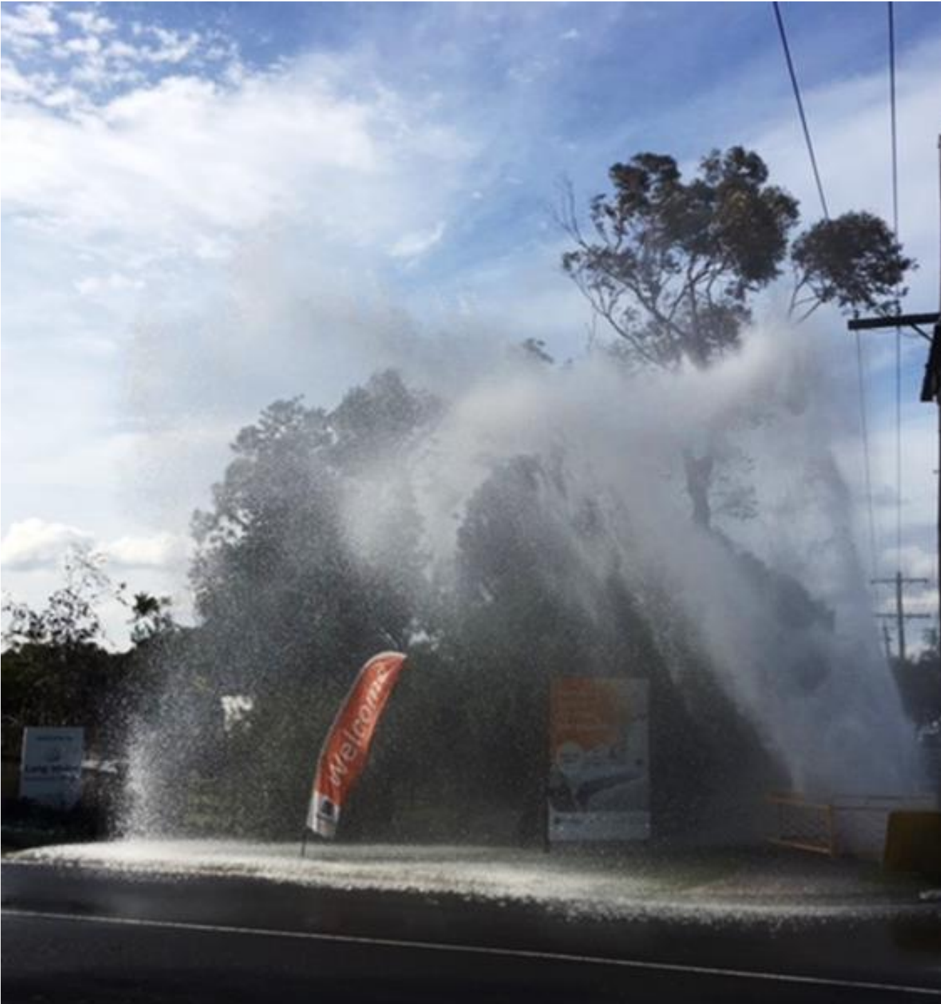
Image shows damage to a water main where the assets were not properly protected.
