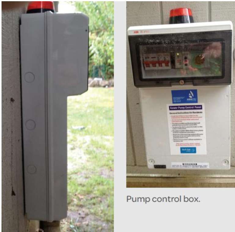
Figure 14 – Pump control box
