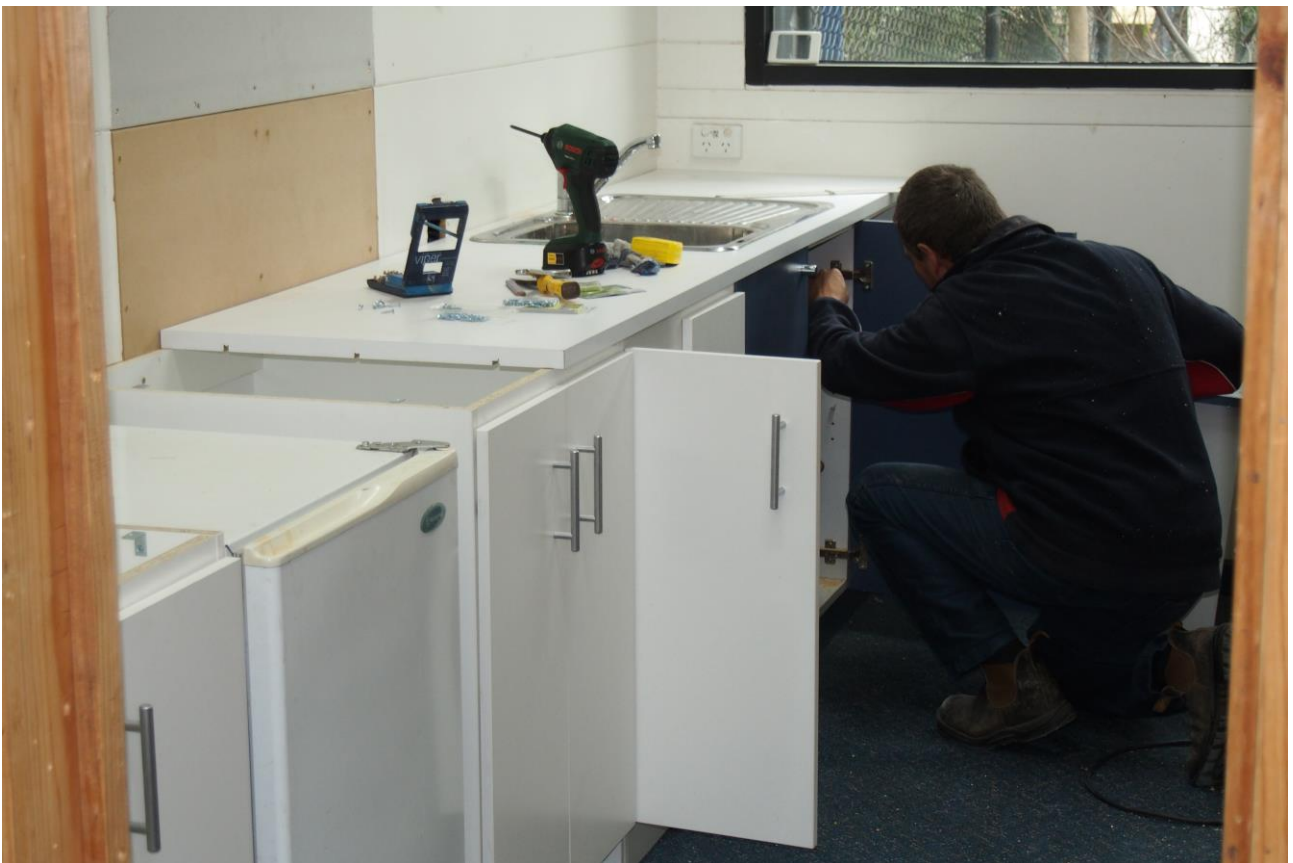
Caption: South East Water builder Bruce installing the new kitchen at McClelland's wellbeing centre.
